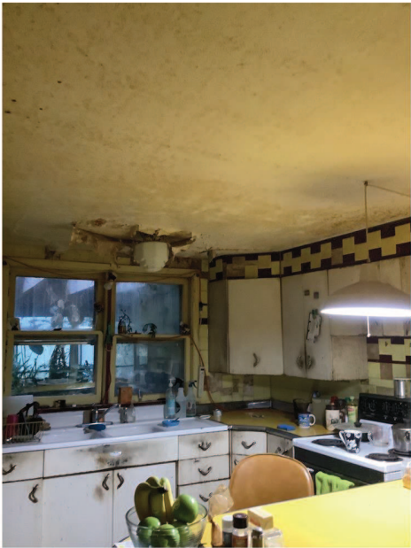
mold on Kitch Ceiling
